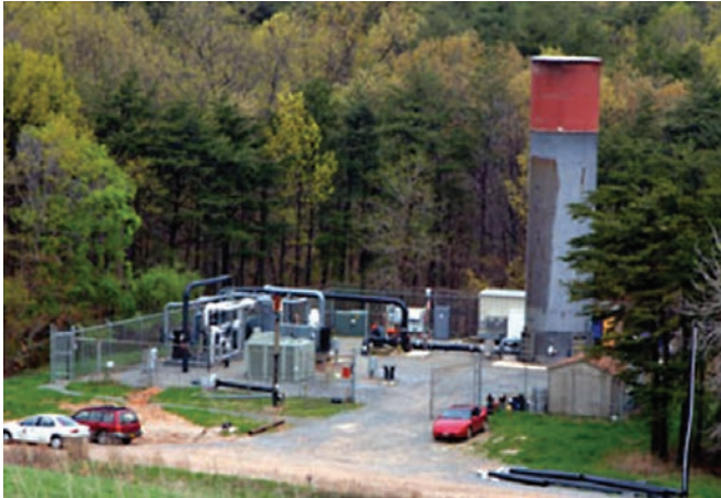
SANDY HILL LANDFILL GAS PROCESSING PLANT (SOURCE: HTTP://WWW.NASA.GOV/MISSION/EARTH/EVERYDAYLIFE/ARCHIVES/0508LANDFILL_PRT.HTM )
