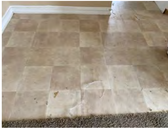
Photo #13: 12" White Square Pattern Linoleum Unit 11 Sample Set #23 – Non-ACM
