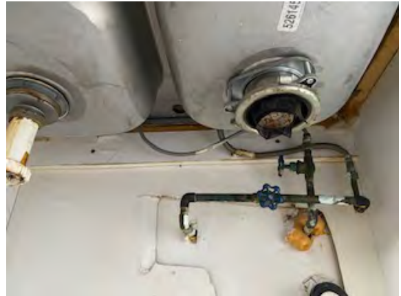
Photo #8: No Sink Undercoat/Insulation Most Units
