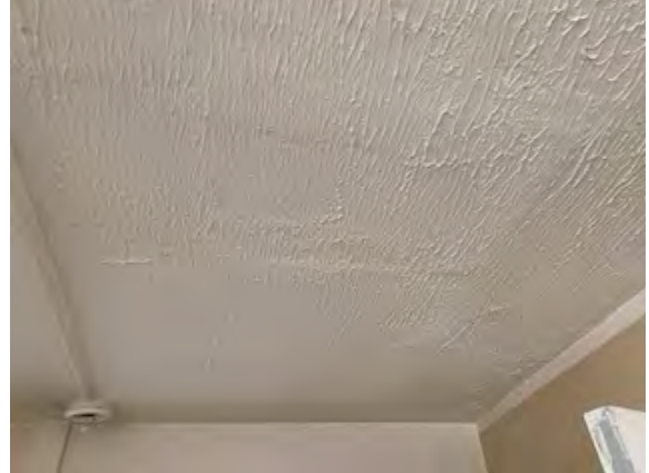
Photo #12: Typical Textured Ceiling 2 nd and 3 rd Floor Units Sample Set #9 – Non-ACM
