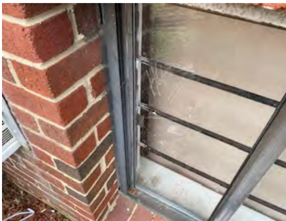
Photo #21: Typical Exterior Window Caulk Sample Set #11 3% Chrysotile Asbestos
