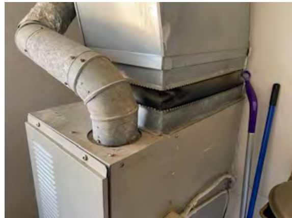
Photo #6: Typical Duct Vibration Damper Kitchen HVAC Units Sample Set #12 - Non-ACM
