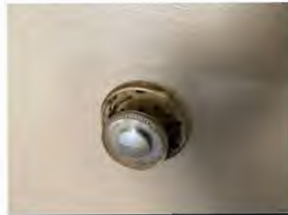
Photo #11: Mercury Thermostat Some Units
