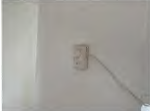
Photo #4: Non Mercury Thermostats Throughout Building
