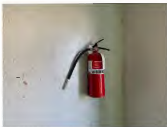
Photo #6: Fire Extinguishers Hallways on Each Floor
