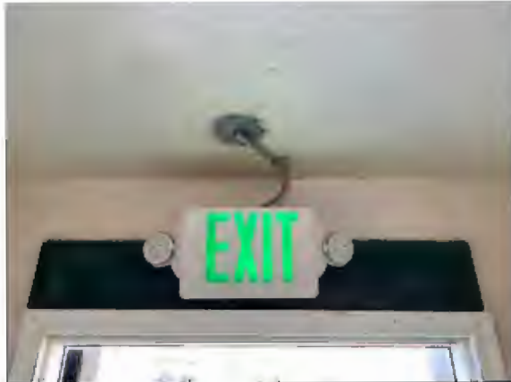
Photo #7: Emergency Exit Lighting Hallways
