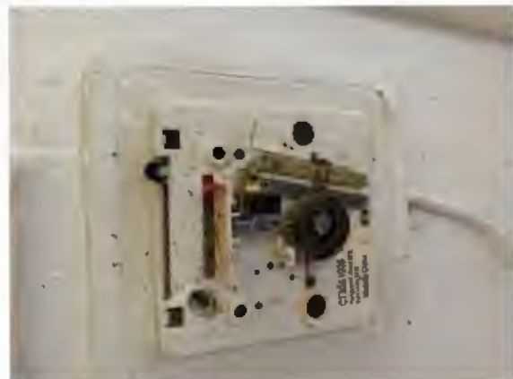
Photo #3: Non Mercury Thermostats Throughout Building
