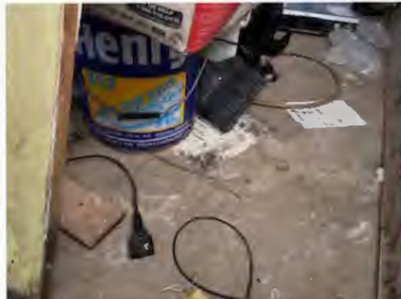
Photo #9: Electric Meter Room 5 Gallon of Roofing Sealant
