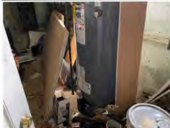
Photo #5: Electric Meter Room 5 Gallon Buckets of Paint
