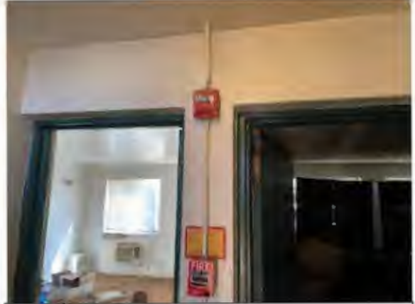
Photo #8: Fire Strobe Lights Hallways on Every Floor
