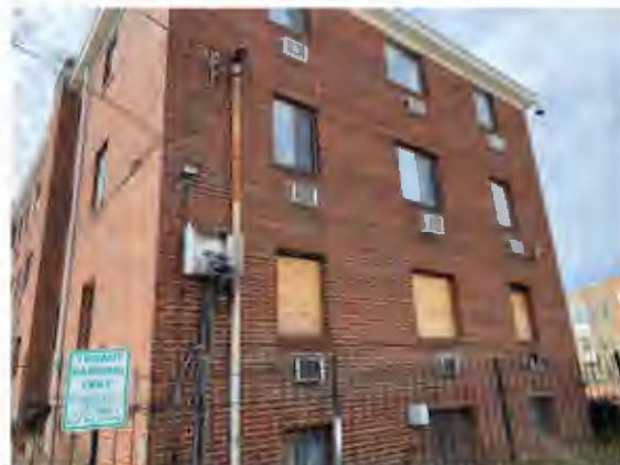
Photo #4: Exterior Window Lintels LBP in Poor Condition
