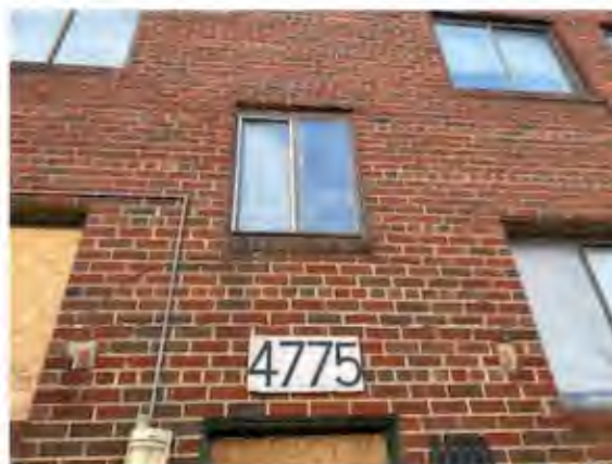
Photo #2: Front Door Jambs Intact LBP
