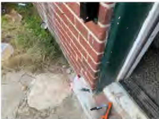
Photo #3: Exterior Door Jambs Intact LBP
