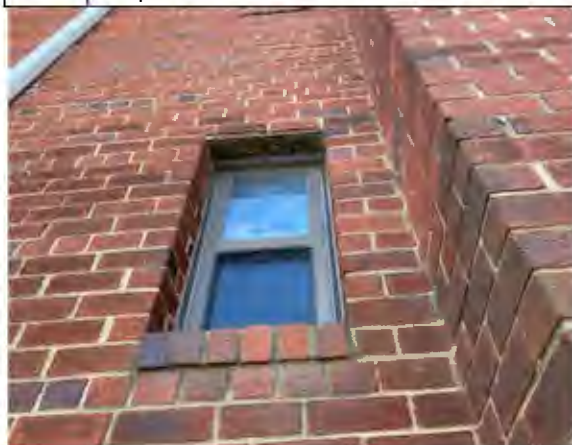
Photo #24: Typical Exterior Window Caulk Throughout Property Sample Set #11 – 3% Chrysotile Asbestos
