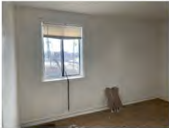
Photo #7: Typical Interior Window Caulk Throughout Building Sample Set #12 – Non-ACM
