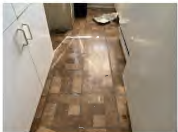
Photo #15: Small & Big Brick Pattern Linoleum & Mastic Unit 8 Sample Set #17 – Non-ACMs
