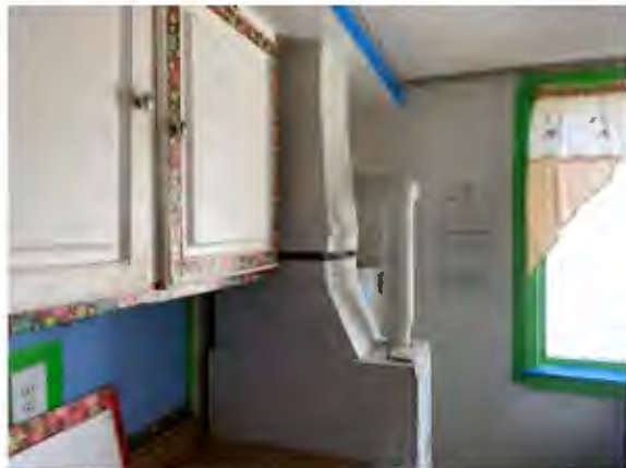
Photo #11: Typical Vibration Damper Kitchens Sample Set #10 – Non-ACMs
