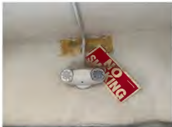
Photo #7: Emergency Lights Hallway
