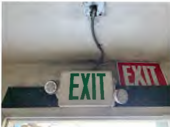
Photo #5: Exit Lights Hallway
