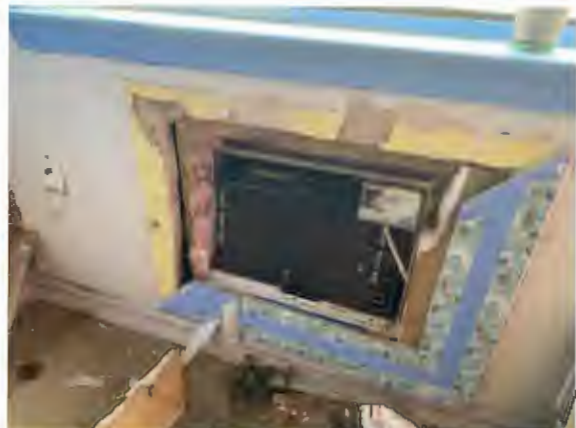
Photo #4: Typical Window Air Conditioning Units Throughout Building
