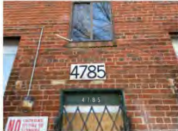
Photo #2: Front Door Jambs Intact LBP
