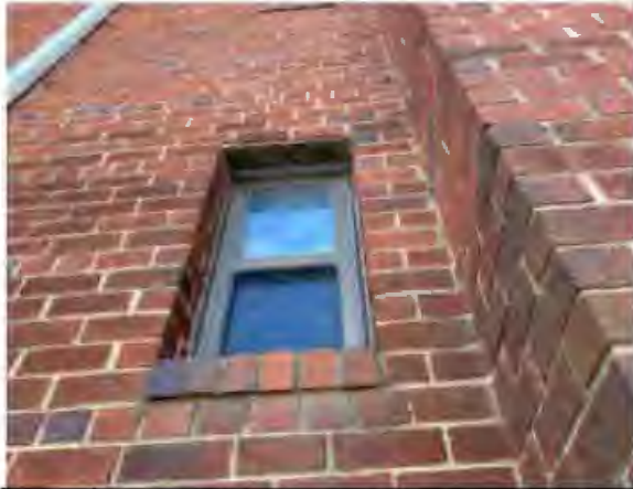
Photo #7: Exterior Window Lintels LBP in Poor Condition
